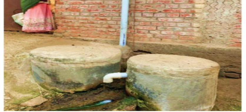
Black water from Single pit
