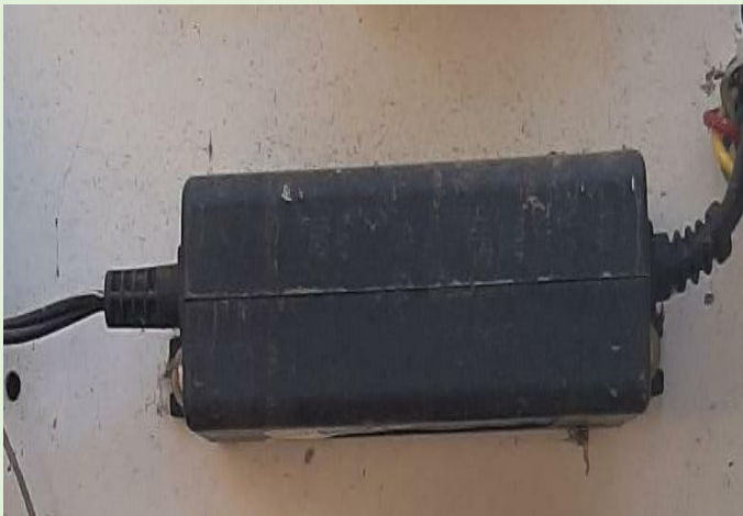
RTU Charging Point
