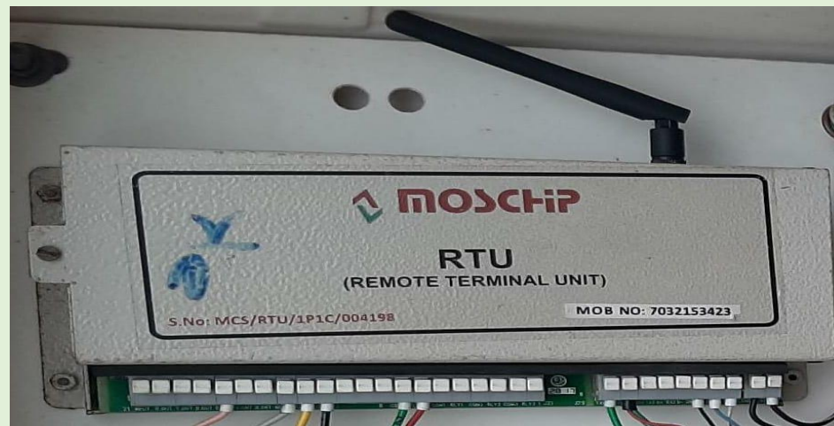
RTU – Remote Terminal Unit ( GSM Sim, Memory Card & Antenna)
