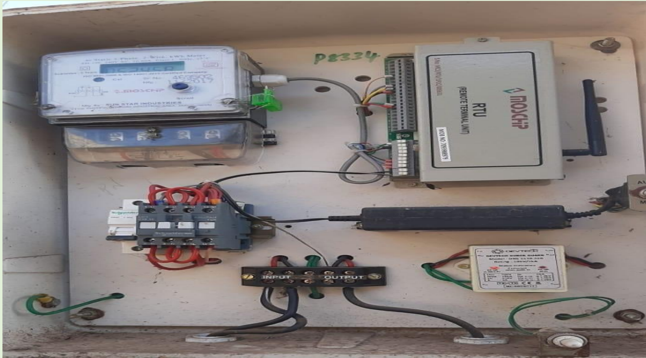
CCMS – Centralised Control & Monitoring System (Junction Box)
